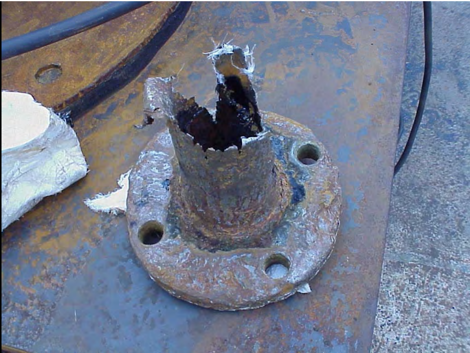
DETERIORATED TANK VENT
