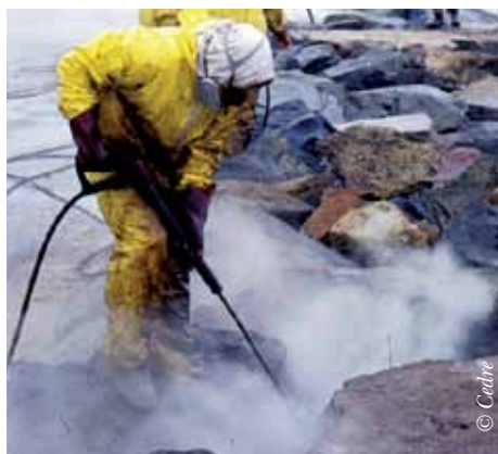
Risks of pollutant splashing
