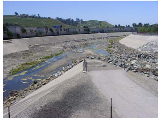
Flood Control—San Juan/Arroyo Trabuco Creeks
