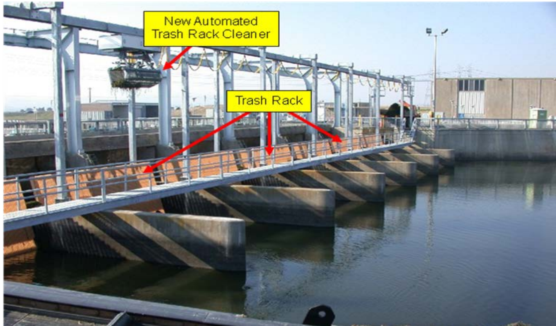
Figure 5. View of the new SDFPF trash rack and automated cleaner.
